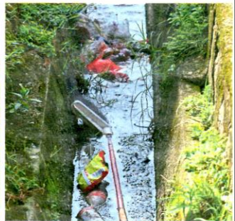
Clogged drains contribute to the foul smell in the area.
