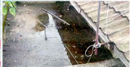
Stagnant water at the rooftop are potential breeding grounds for mosquitoes.
