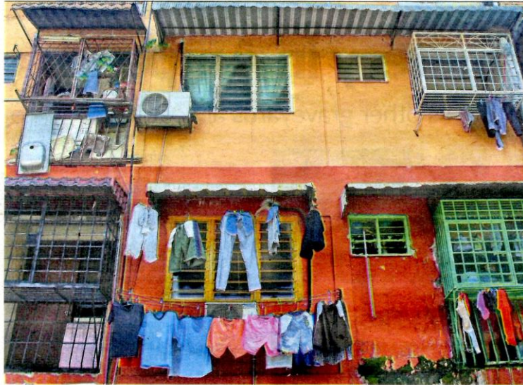
The poor collection of maintenance fees contribute to the unkempt surroundings.
